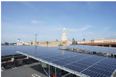
Carport-type solar power generator for captive consumption (Aimi Premium Outlets)
