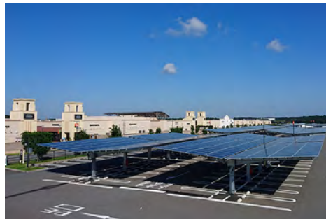
Carport-type solar power generator for captive consumption (Shisui Premium Outlets)
