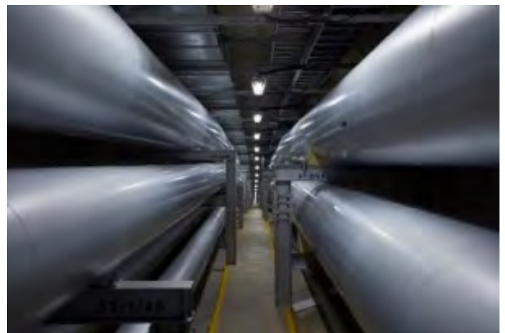
Underground heat supply piping
