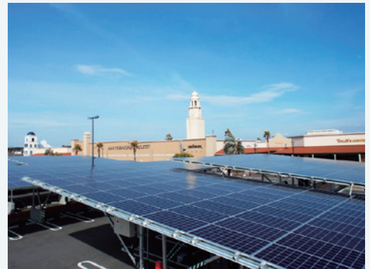
Ami Premium Outlet's carport-type solar power generator for captive consumption
