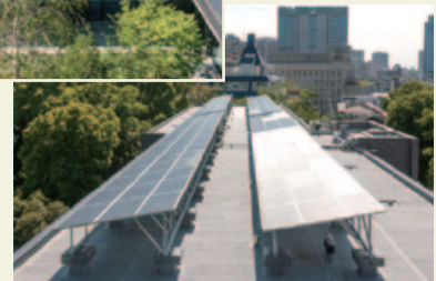
Solar power generation
