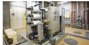
Sewage and water pumping facilities for emergency disasters
