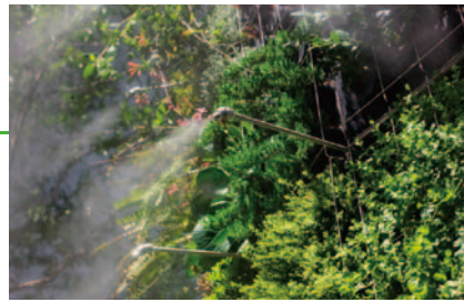
Micro-misters Water is automatically sprayed in an ultra-fine mist when the temperature rises, cooling the surrounding air temperature as it evaporates.
