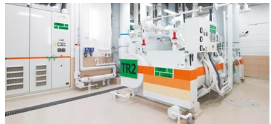
Inverter turbo chiller:
